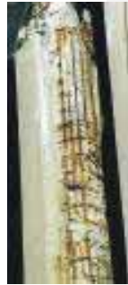
Deterioration of concrete due to improperly designed rebar splices and lack of reinforcement, often leads to premature splice failure.
