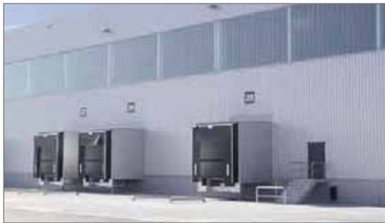
Installed on wall.
